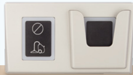
Energy saver + Room status selection, wall-mounted inside the room. (DINES + DND)
